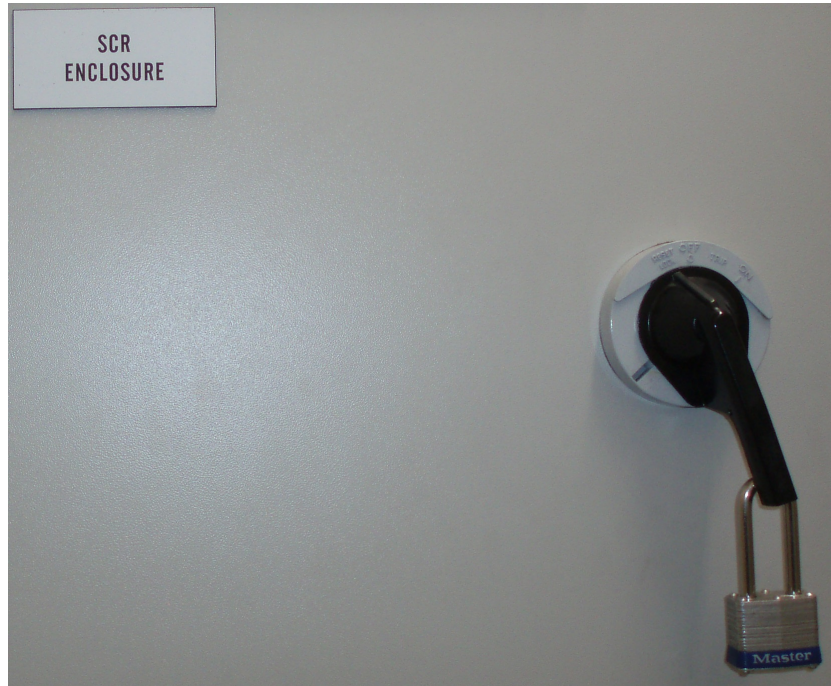
Figure C.2: SCR enclosure and the padlock.
